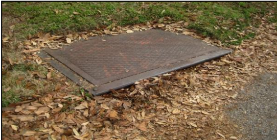
Clogged catch basins cause street flooding
